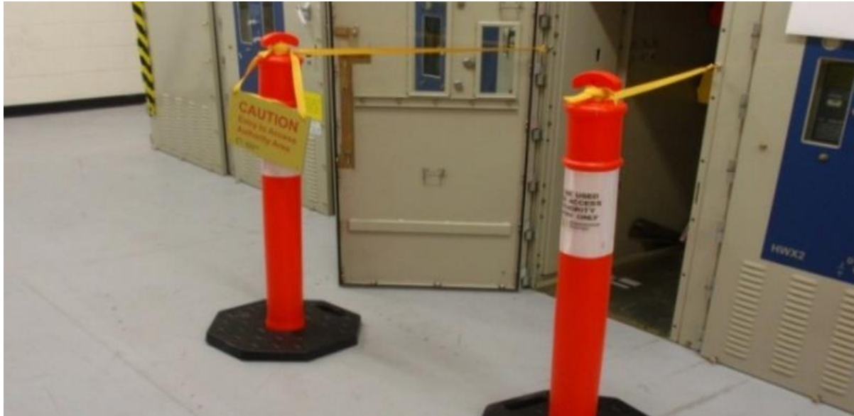
Figure 5. Example of switchgear under Access Authority with the Yellow Tape-In Method defining the entry area. Refer to Clause 7.7.4 Descriptions of barriers and signs for correct signage.
