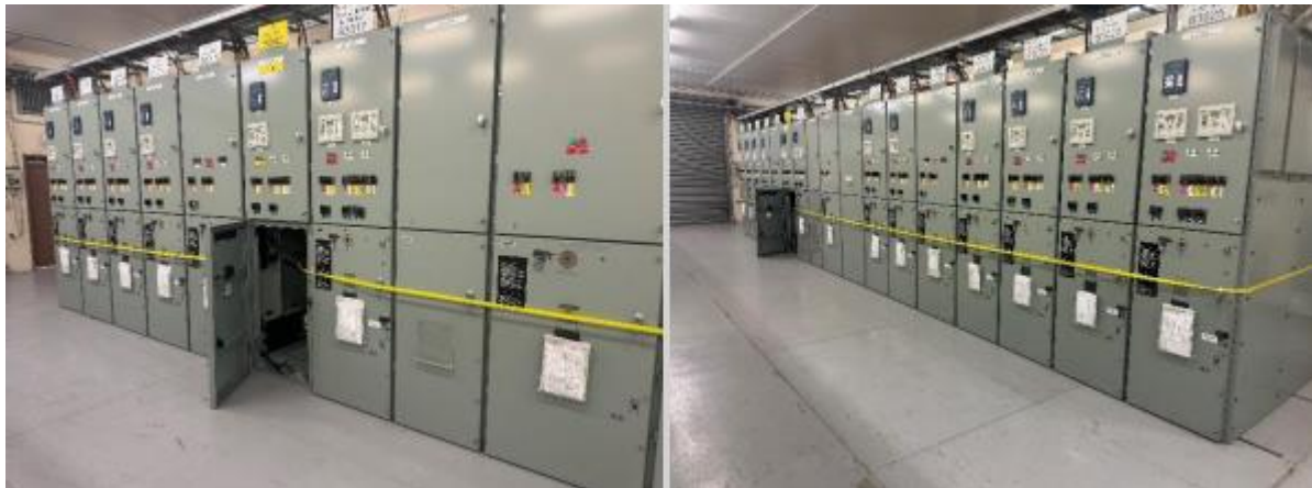
Figure 6. An example of the Yellow Tape-Out Method used on indoor metal-clad switchgear
