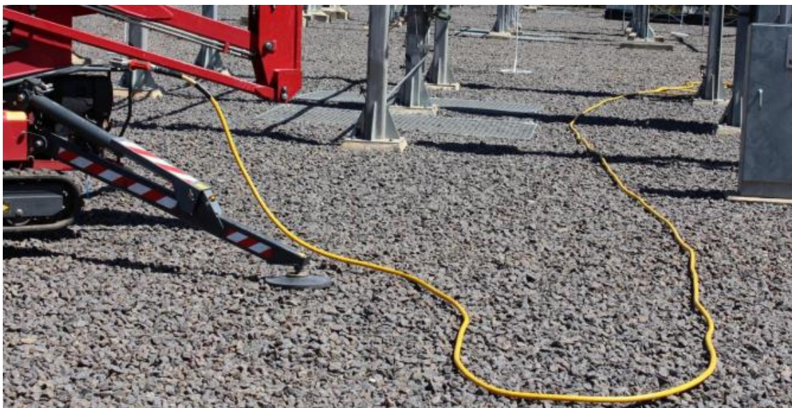
Figure 10. EXAMPLE OF VEHICLE EARTHING IN A ZONE SUBSTATION
