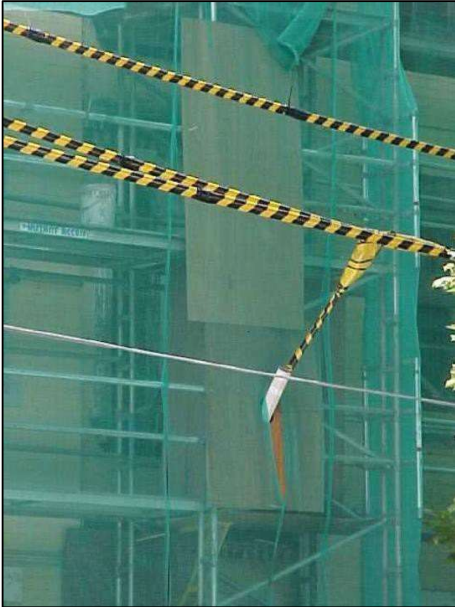
FIGURE 4. LOW VOLTAGE ELECTRICAL WIRES PASSING THROUGH A SCAFFOLD.
